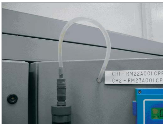
Figure 9: Cation exchange column connected by silicone rubber tubing.
