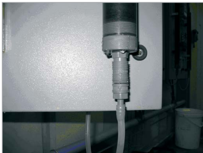
Figure 10: Lower end of column with leaky silicone tubing.
